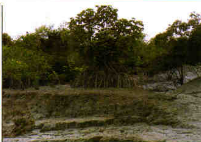
Land slide due to creek erosion
